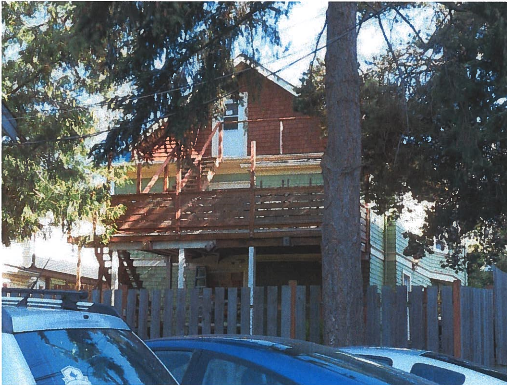
View of the south elevation with the staircase and door to be removed
