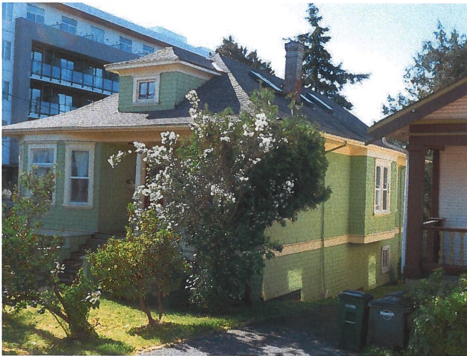
Northwest view of the house – three new skylights on the west-facing roof
